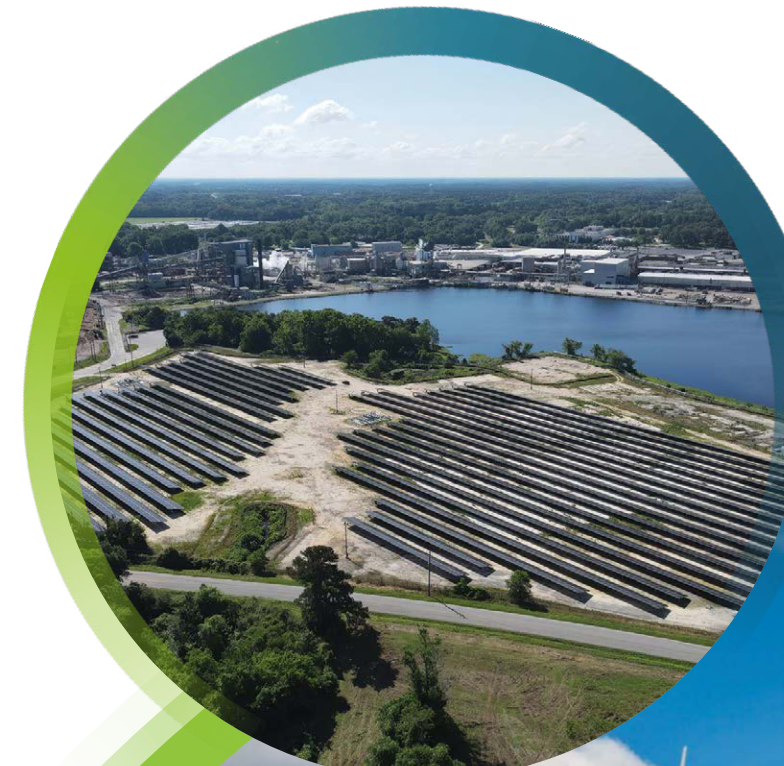
Solar Panel Farm, Corporate Headquarters, Hartsville, SC
